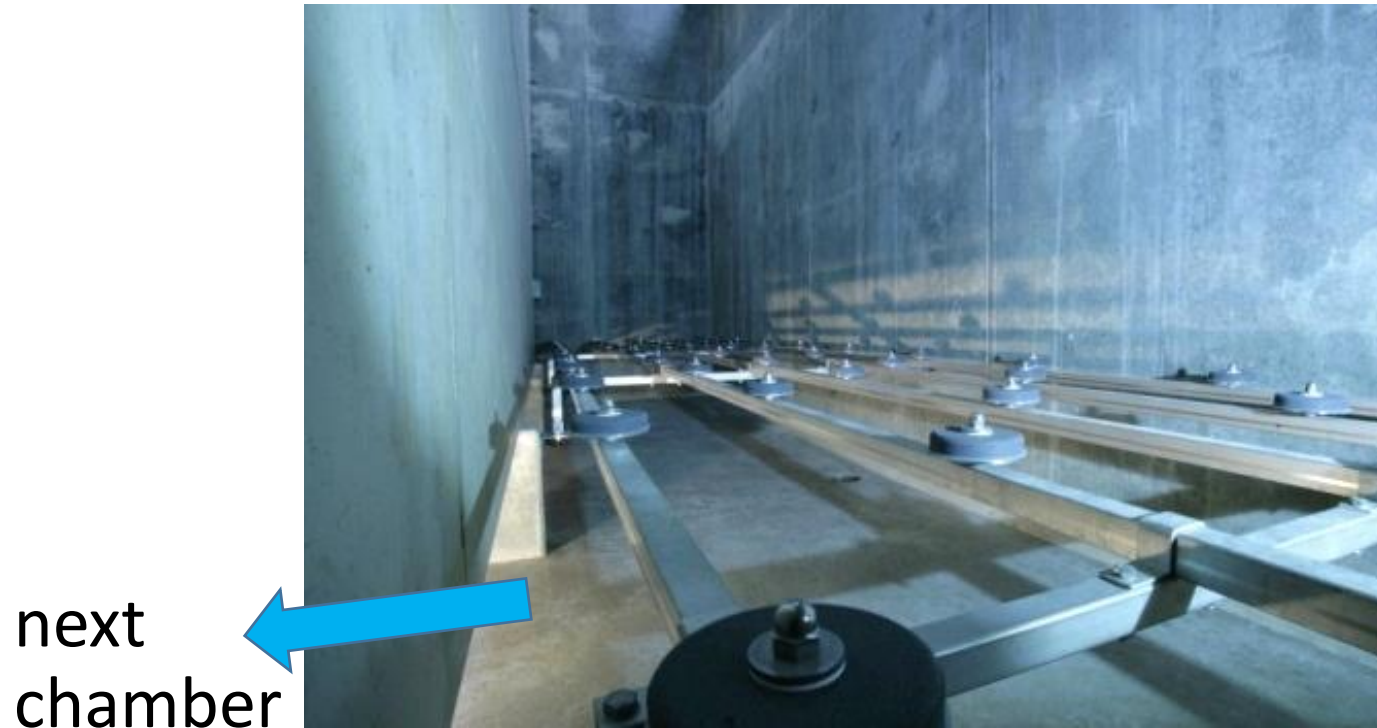
ozone injection chamber with ceramic diffusers
